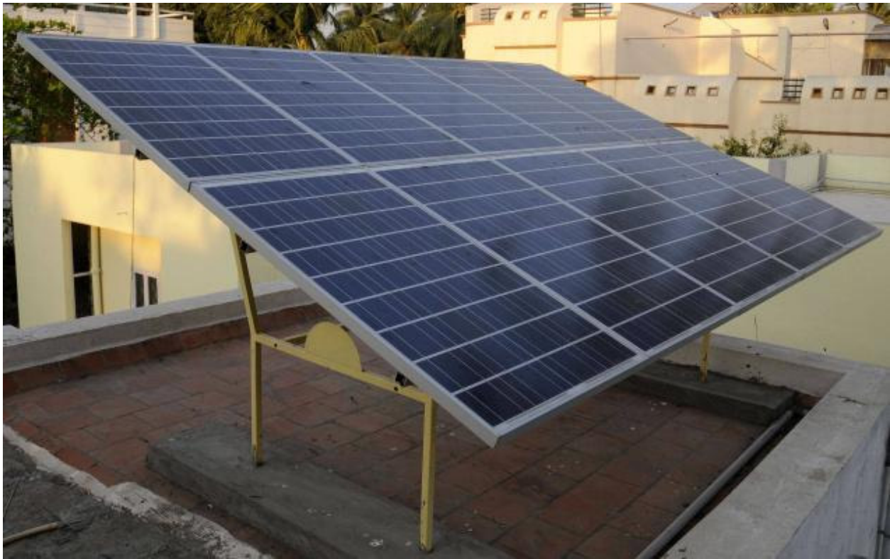
A typical roof top photo voltaic solar system
